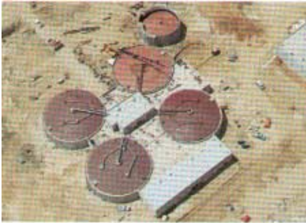
Four 90 Foot diameter Walker Process Fixed Covers each with three 48 inch Gas Lifters at Dallas, Texas, South Side WWTP, also shown, is one 60 foot diameter spiral-guided Gasholder.
