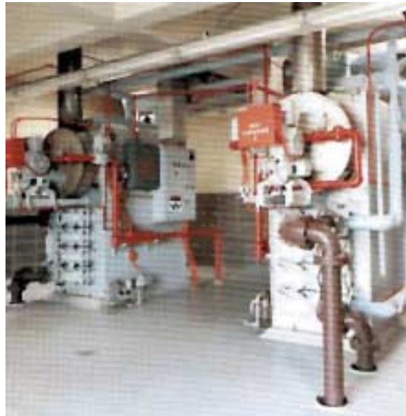
Above, two 750,000BTU/hr. EB HeatX units at Hinsdale, IL. Picture taken from the burner side.
