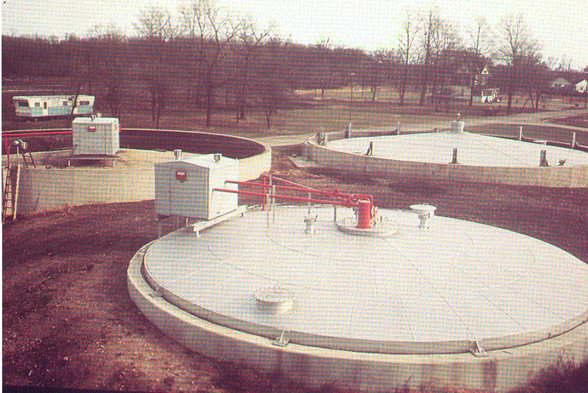
At DeKalb, Illinois a Fixed Cover and Floating Cover with GasLifter mixing in each, The secondary cover in the background is a Walker Gasholder.
