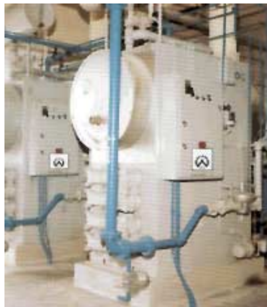
Below, the picture shows the boiler viewing port at the opposite end from the burner.
